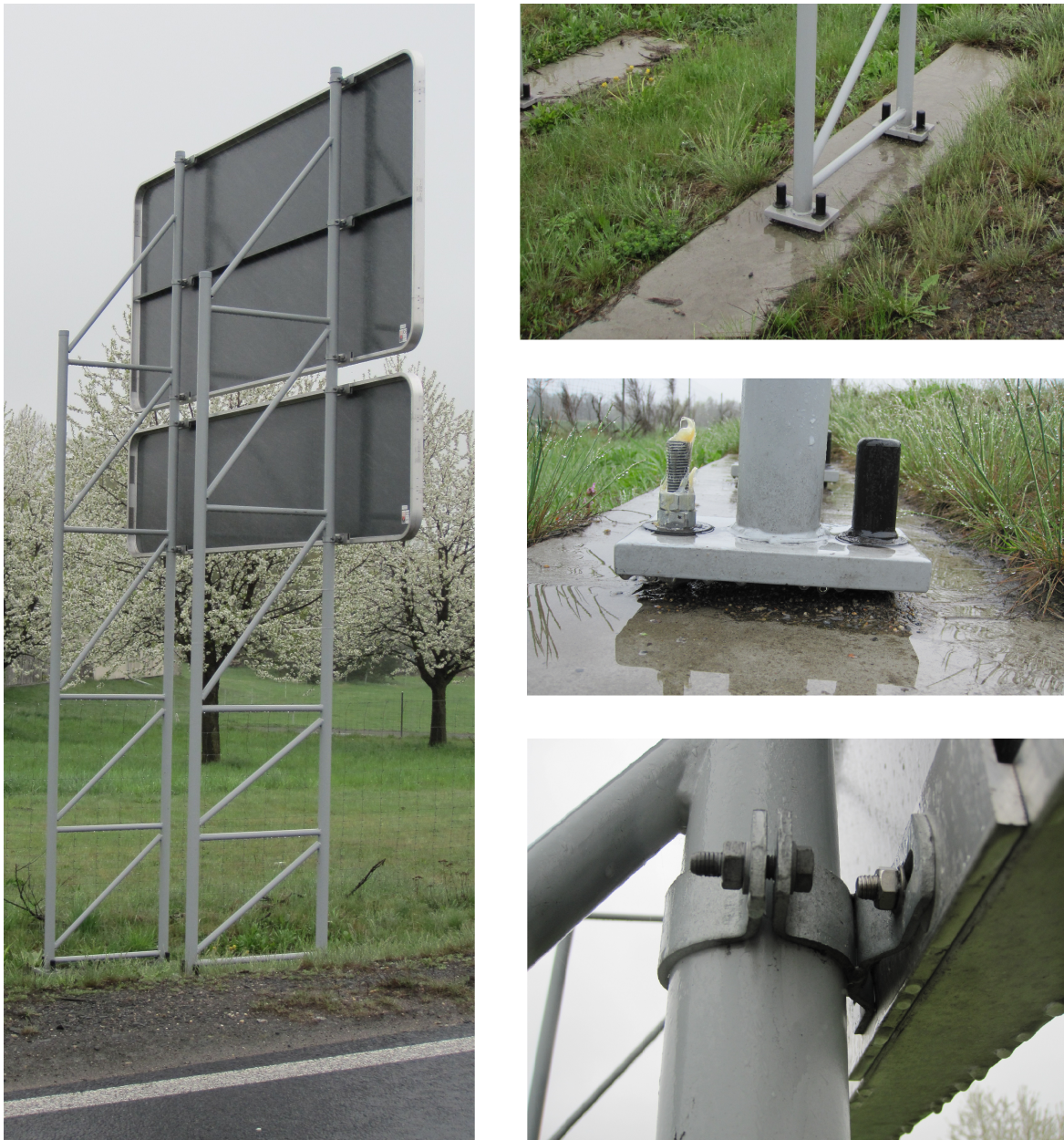
Figure A.1: Pictures of a typical structure Left: typical traffic sign support structure. Right: details. Upper: rigid, concrete foundation. Middle: base plate bolted on the foundation. Down: connection between truss and sign.
